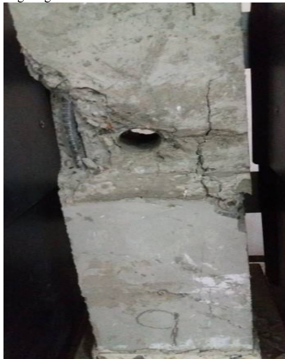
Failure mode of column, Fig # 02.
