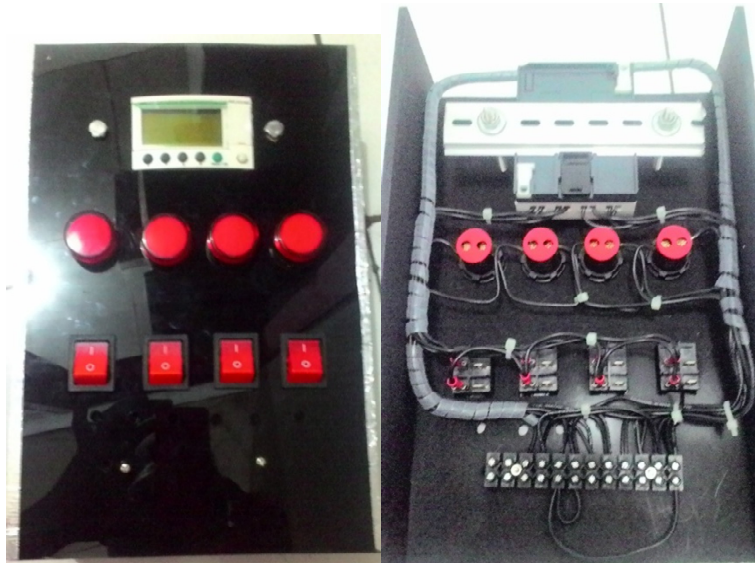
Figure 3.2 Temperature Display Control Panel space Source: Personal Documentation
