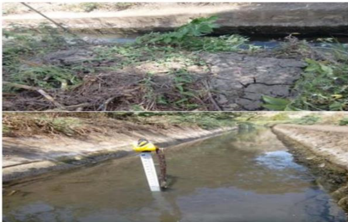
Figure 20. Sediment deposition in irrigation canal
