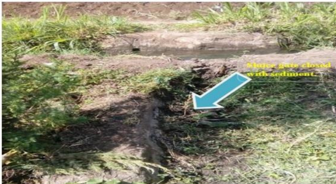
Figure 21. Damaged gate and closed sluice gate
