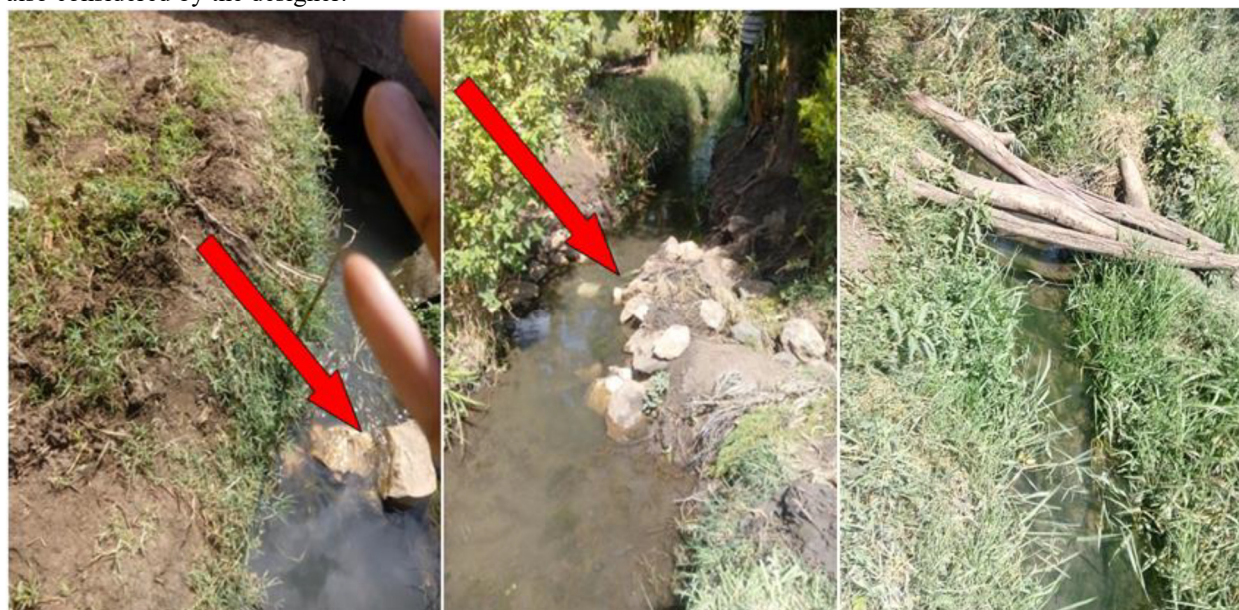
Figure 23. Cross road problem through the canal
