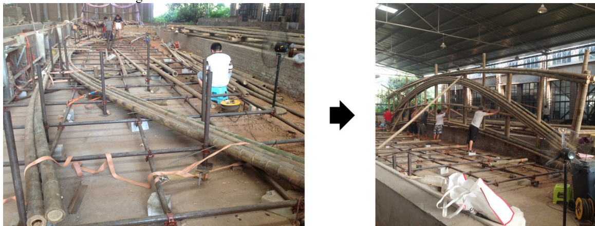
Figure 2. Bamboo arches bent using steel scaffolding as the Cartesian system for reference. The truss was erected manually by workers. Photographs: Daniel Stamatis.
