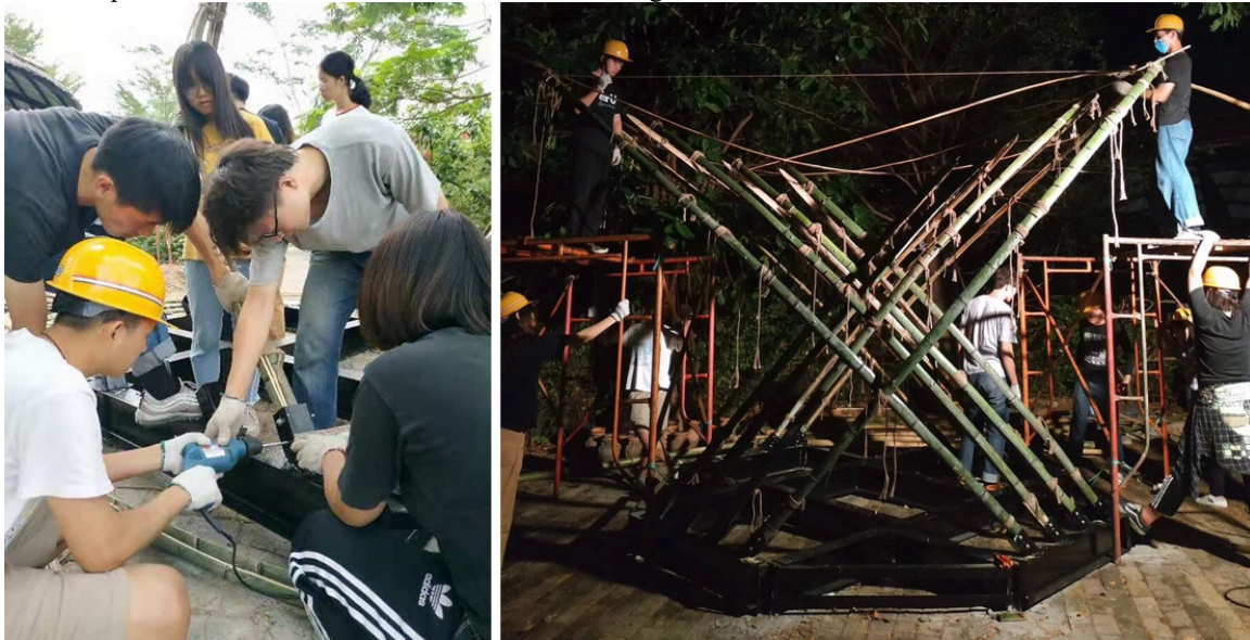
Figure 12. Installation of the eight arches on the metallic base. Photographs: Chen Yudie and Li Meishuang.
