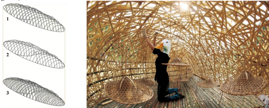
Figure 1. Weaving bamboo in the interior of the shelter after three layers of split bamboo arches. Created by Zhong Wenzhou, Ma Danhong, and Zheng Xing.
