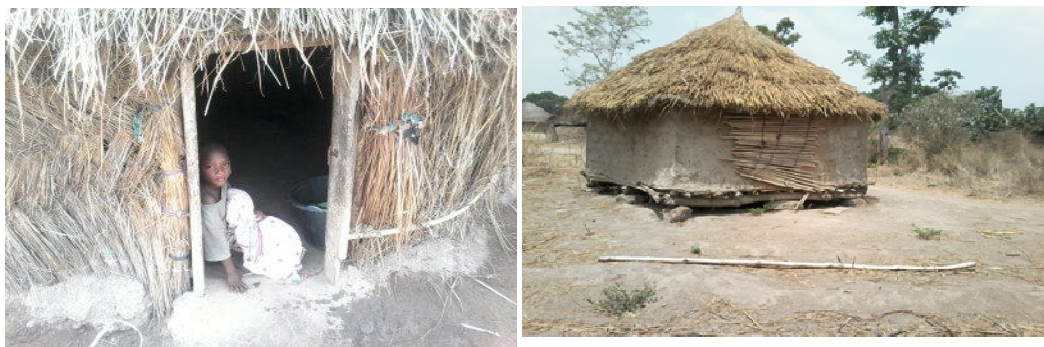
Plate 6: Door and Window Conditions of Fulani Housing at Iyana-olomi, Ogbomosho South Local Government Area, Ogbomosho. Source: Author's Fieldwork, 2015
