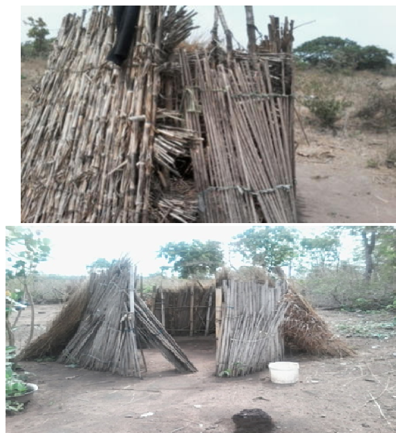
Plate 8: Outdoor Bathroom facilities at Gaa Iyelu I, Surulere Local Government Area, Ogbomoso. Source: Author's Fieldwork, 2015
