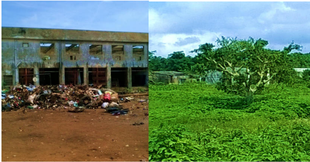
Plate 2: Uncompleted Abandoned Structure Turn into Refuse Dumps in Tanke Area. Source: Author's Field Survey, 2015
