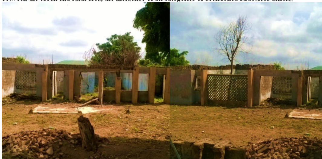
Plate 1: Uncompleted and Dilapidated Abandoned Structures in the Odota.
