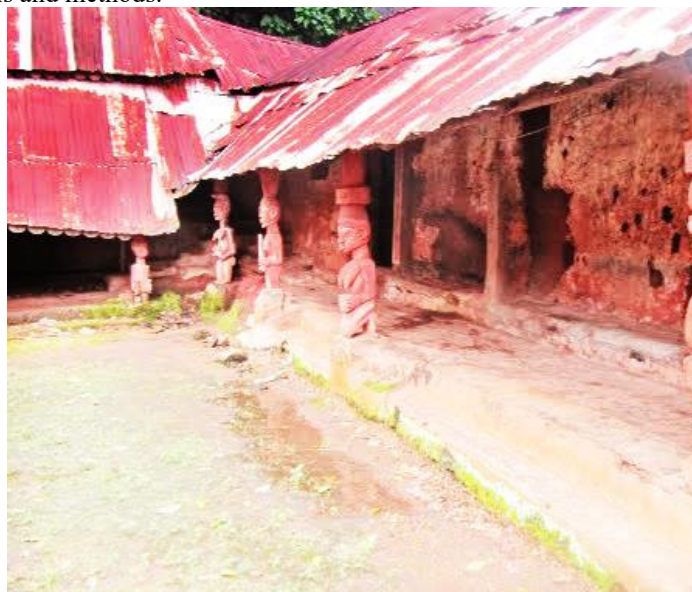
Plate 6: Abandoned Yoruba vernacular architecture at Idanre town, Ondo state, Nigeria. Source: The Sun news, 2018
