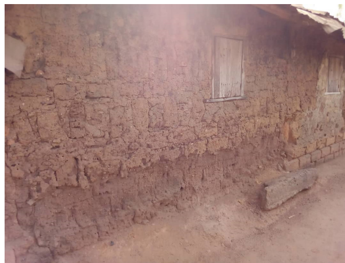
Plate 2: Abraded surface of a wall constructed with laterite: Authors Field work, 2019
