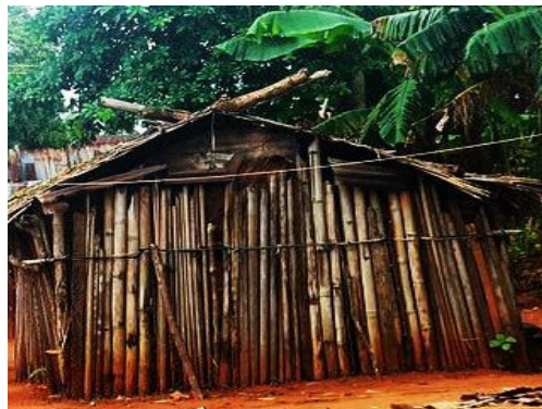
Plate 5: Effect of incessant rainfall on bamboo wall. Source: Adekunle et al., 2008.
