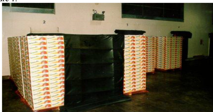
Figure 1: A commercial forced-air cooling system (Source: FAO 2002).
