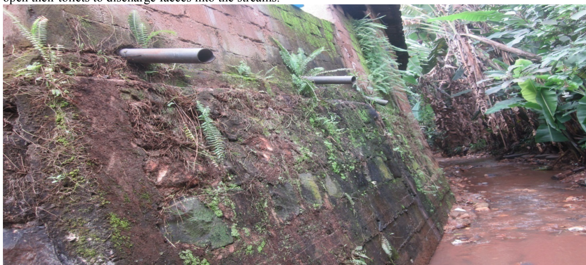
Figure 2.0. Pipes projecting from a toilet into a nearby stream in New layout Nkwen. Picture by Polycarp Ndikvu July 2015 (Figure 2) and thick film, of stool settles after the rains (figure 3).
