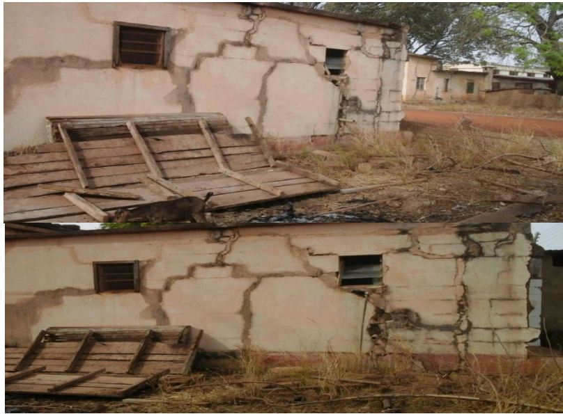
Figure 1. Staff bungalows at Navrongo College of Education built with sandcrete blocks developing multiple cracks due to high diurnal temperature.
