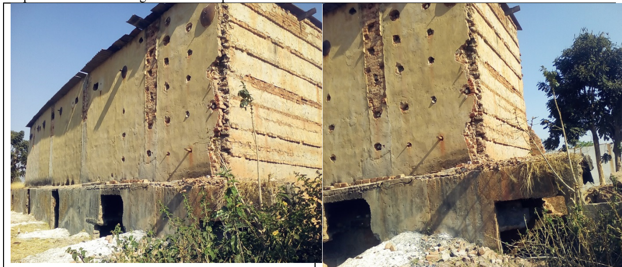
Plate 2: Dilapidated tobacco barns at Camperdown Farm in Mt Darwin.
