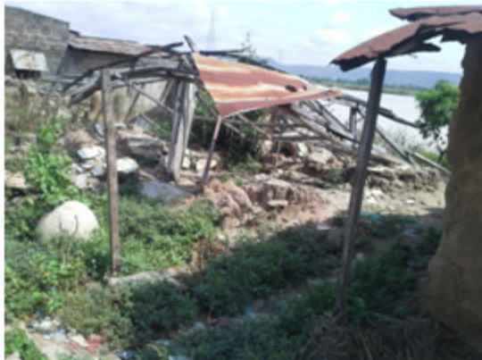
Figure 1.1: Showing collapsed shelter by the riverside Source: Author's fieldwork 2013
