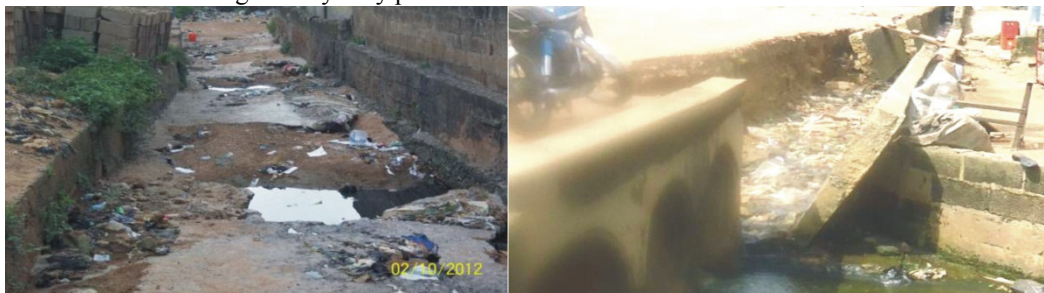
Plate 5: Showing dilapidated & damaged drainage System in the study area
