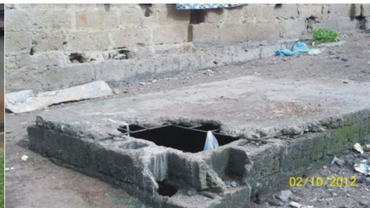
Plate 4b: Showing dilapidated Septic Tank Source: Field survey, 2012
