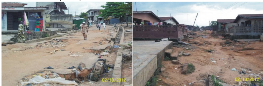
Plate 8: Condition of Access roads in the study area
