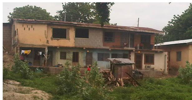
Plate 1: Example of dilapidated building identified in the Area
