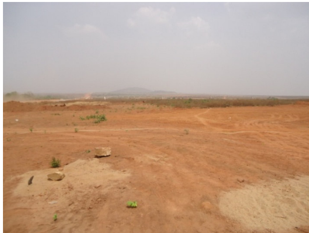
Plate ii: Bare surfaces resulting from construction activities in Chinka, May, 2013
