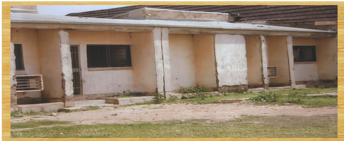
Plate 8: Picture showing part of a poorly maintained building in Abdusalam Housing Estate. Source: Authors' field survey, 2015.
