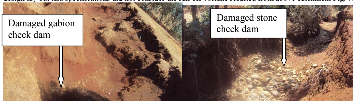
Figure 7. Ineffective stone and gabion check dams on large gullies.
