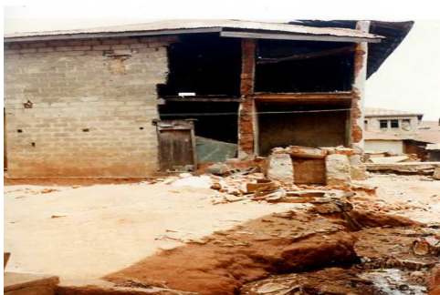
Derelicts Houses in Bere; Lack of Drainage And Appropriate Waste Water Disposal.
