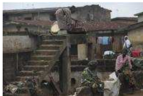
level of housing deterioration
