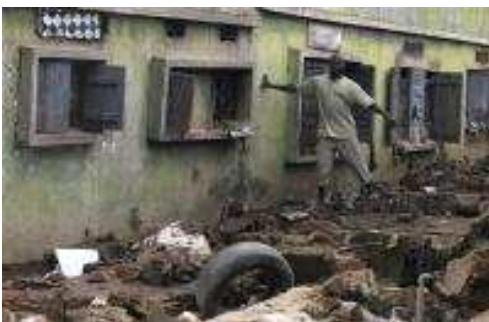
Dilapidated house in Ibadan
