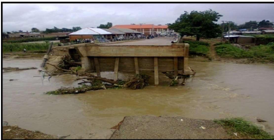
Plate 4.11 Collapsed Shendam Bridge Source: (Buba Y. Alfred 2012)
