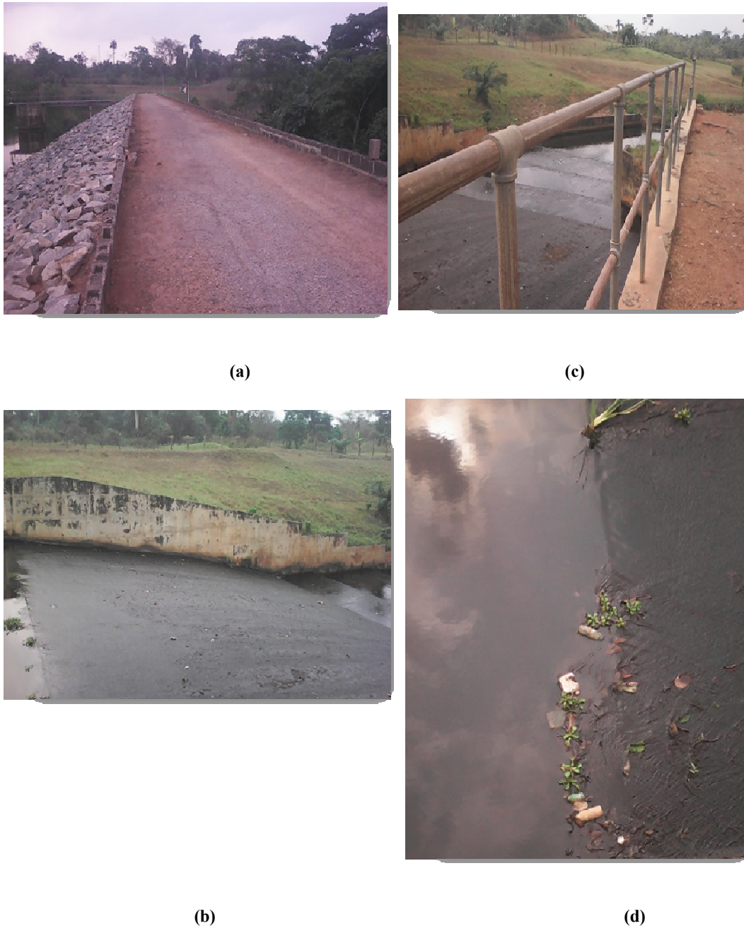
Figure 7: Different section of the dams (a) the crest, (b) side view of the spillway, (c) and (d) section of spillway with debris from upstream.
