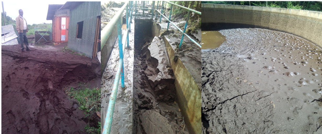
Figure 6: Sedimentation effects at Asella town drinking water reservoir
