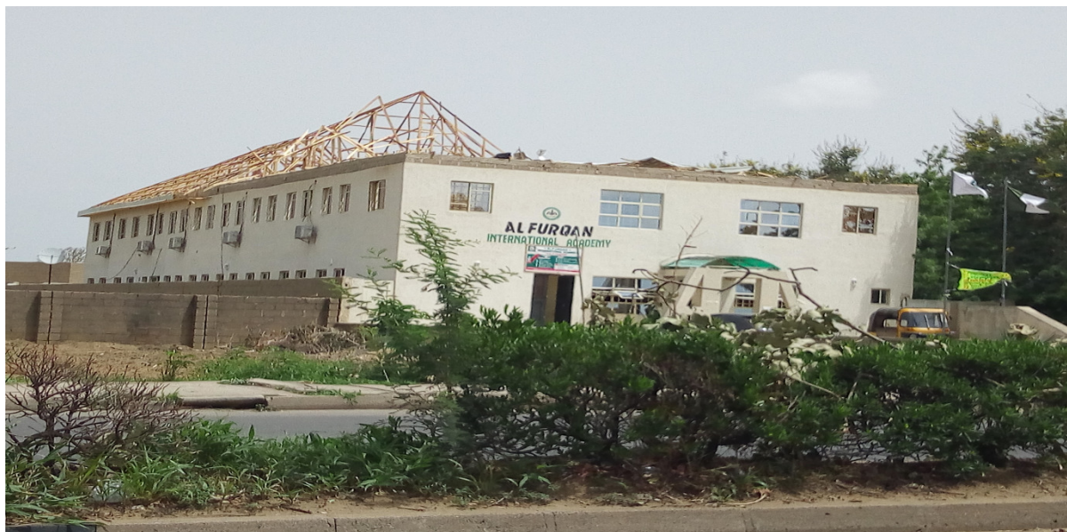
Plate 1: Uprooted roof of Alfurqan International Academy along Abubakar Tafawa Balewa Road, Bauchi Source: Researchers' Field Observations, 2018
