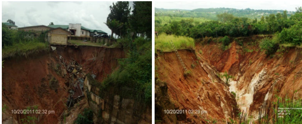
Figure 5: Court house destroyed by gully erosion at Afikpo South LGA
