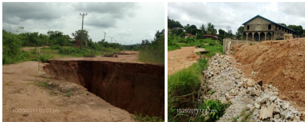
Figure 7: Electric poles and wires under threat by gully erosion at Nguzu Edda and catholic Church fence destroyed by flood water
