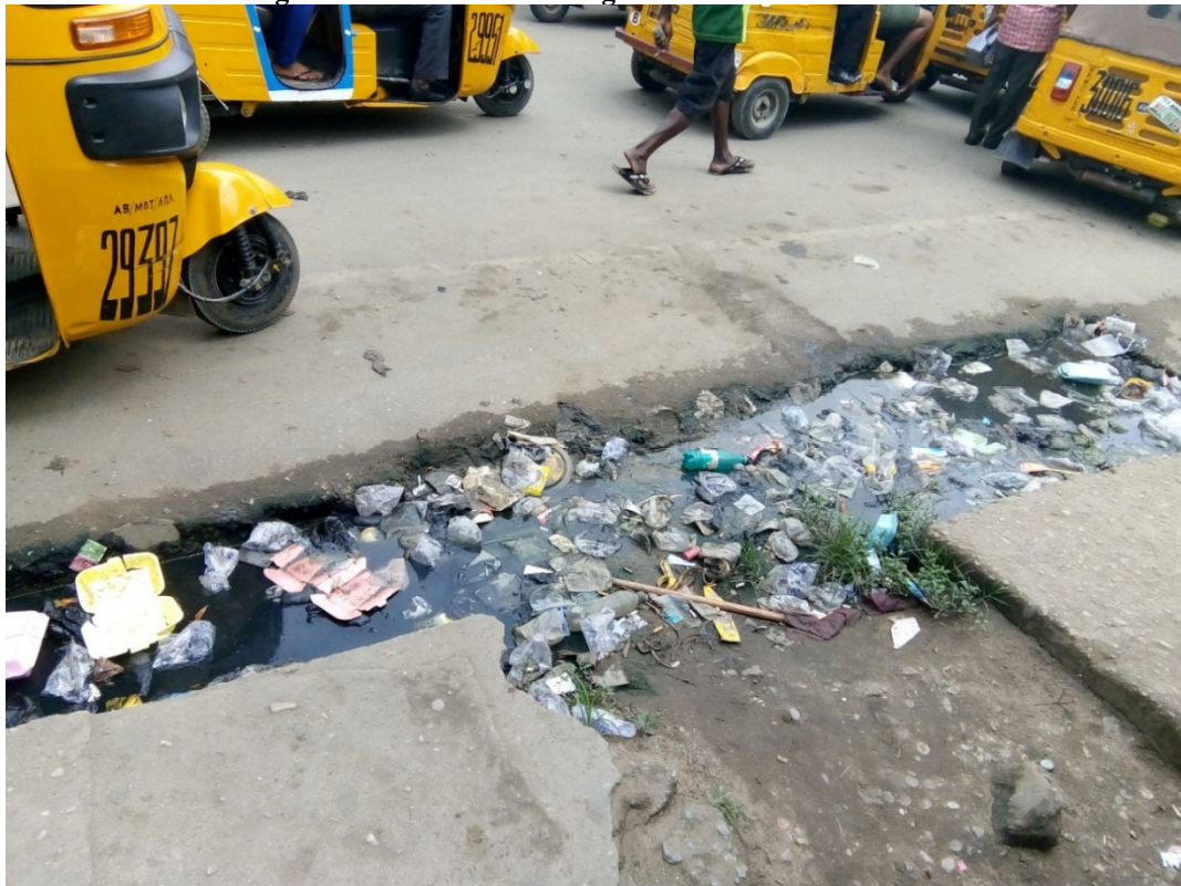
Figure 5: A Refuse-blocked gutter near Aba Main Park
