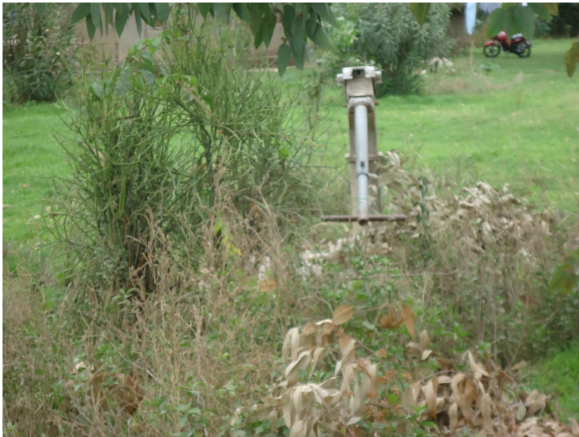
Figure 18. Non-functional shallow well, Dorebafana, near Mekane Eyesus Church.
