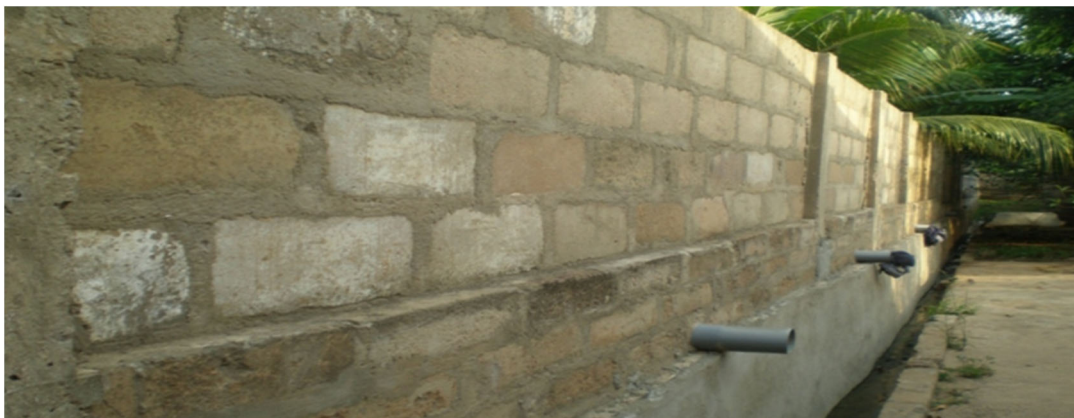
Plate 3.3: Fence wall in Santa Maria to prevent flood water from entering house.
