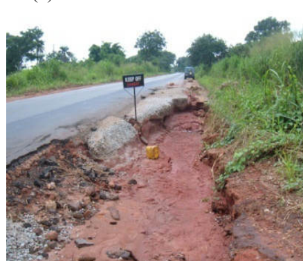
Plate 2 : Pavement conditions at some Locations on Irrua - Auchu road
