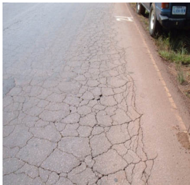
(c) CROCODILE CRACKS AT CH.20+000
