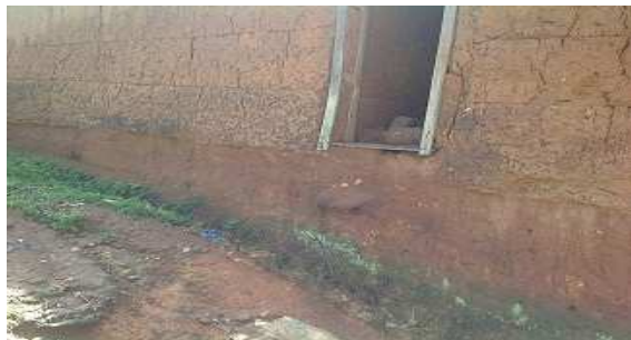
Plate 7: Laterite adobe walls used in residential building constructed with Ilaramokin.. University of Technology,
