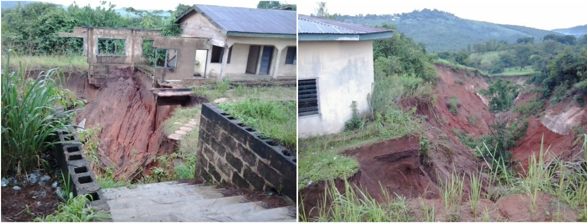
Figure 8. Omagba Gully site.
