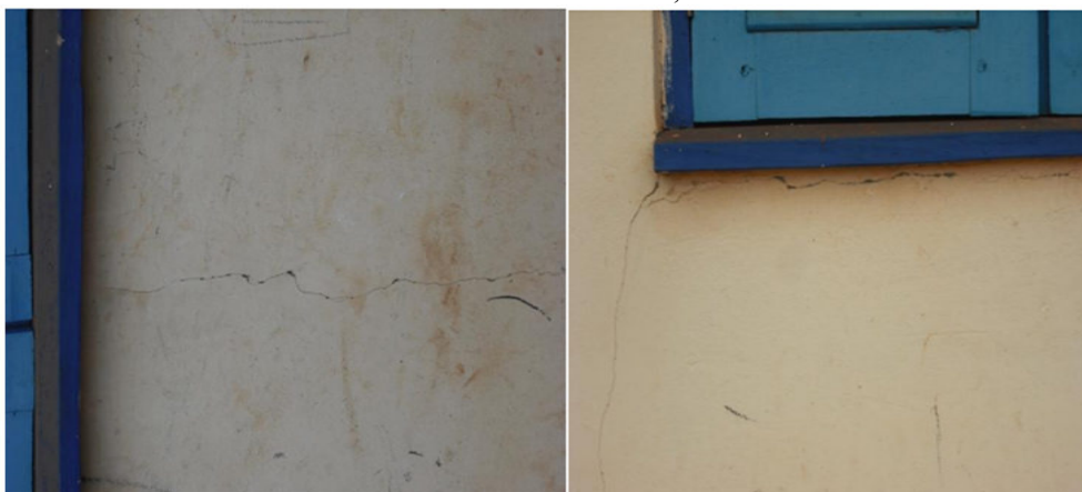
Figure 4: Cracks on some buildings in Kenyasi No.1 due to blasting by Newmont Source: Fieldwork, 2011
