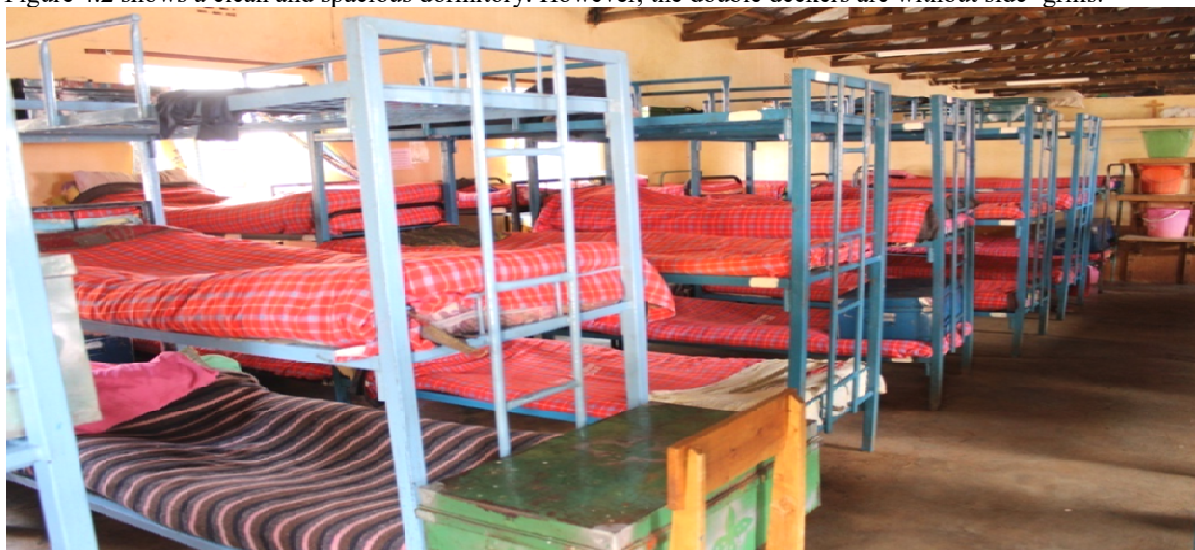
Figure 4.1: An Example of a Congested Dormitory with Triple Deckers with Weak Front- Grills
