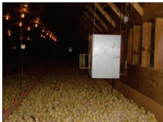
Figure 1: Forced air furnace used for heating poultry house [11].
