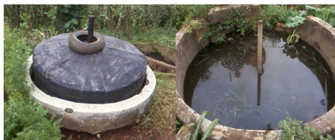
Figure 5.2.1 Common problems with biogas plants in Western Kenya; low biogas production/gas leakage (left) and structural collapse (right)
