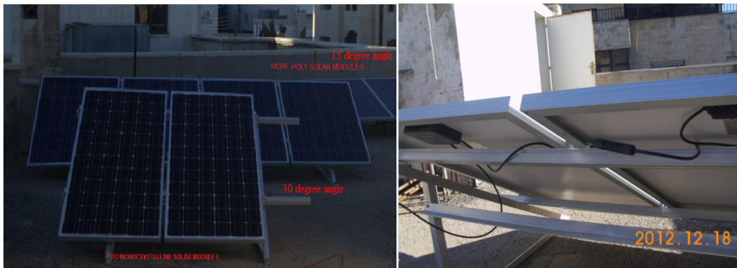
Figure 3. Ground mounting of PV panels by two tilts angle.
