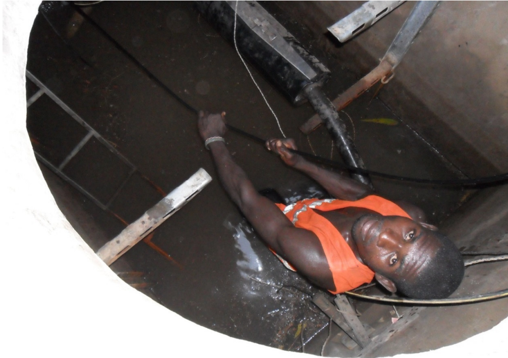
Picture 2: A fiber cable being deployed in an existing tunnel by Vodafone Ghana
