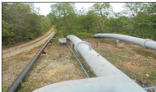
Figure 2. Crude Oil Pipeline Unloaded from SPM
