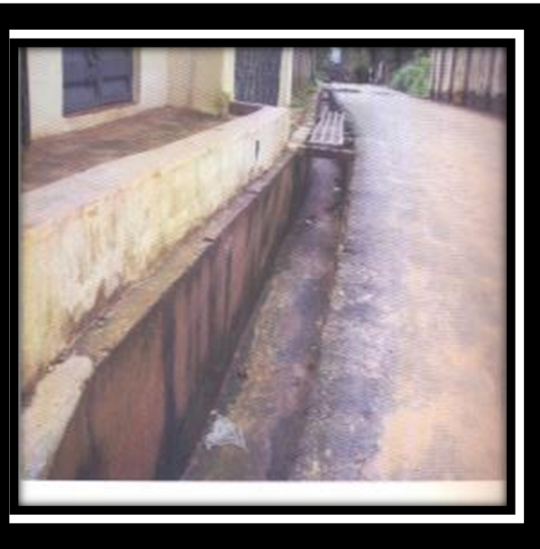
PLATE 7: Building Encroachment on Drainage Source: Anierobi (2010).
