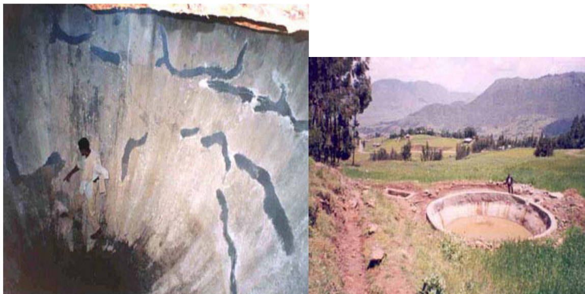
Figure 5 Cracks in the water-harvesting structure (left) (photo H. Rami, UN-OCHA, Oct. 2003) and Leaking from outside (right) (Rami, 2002)
