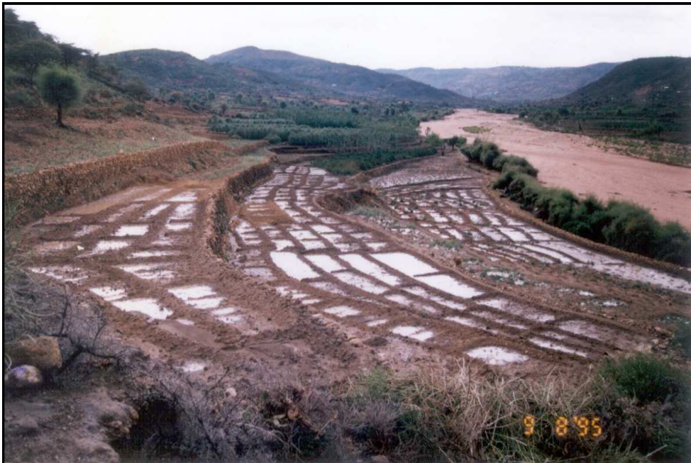
Figure: 3 A typical water harvesting structures constructed for rehabilitating denuded areas in Hararge, East Ethiopia (Dereje, 2006)
