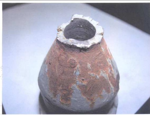
Figure 1: Failed Reducer Nipple
