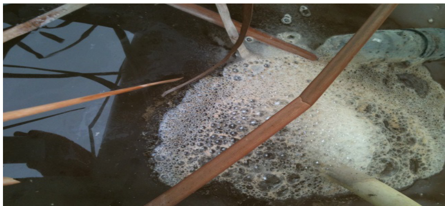
Fig. 6: Foaming formation as a consequence of the rising gaseous nitrogen (outlet RALBI 1 )
