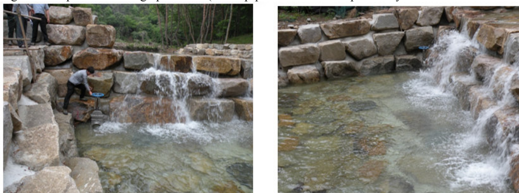
Figure 4. Structurally Improved check dam ( \Phi 300\text{mm} drainage valve and half way fresh water overflow).
