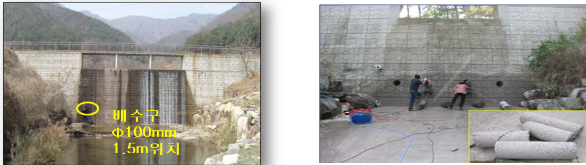
a) Front and side view of non-permeable dam b) Front and side view of dam with structural improvement Figure 1. Example of on-going structural improvements of non-permeability Erosion Control Dam via drilling of four drainage holes.
