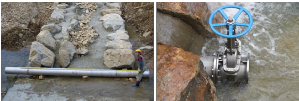
Figure 3. Improved drainage practices (water pipe \Phi 100\text{mm} \Rightarrow replaced by \Phi 300\text{mm} at the base area)
