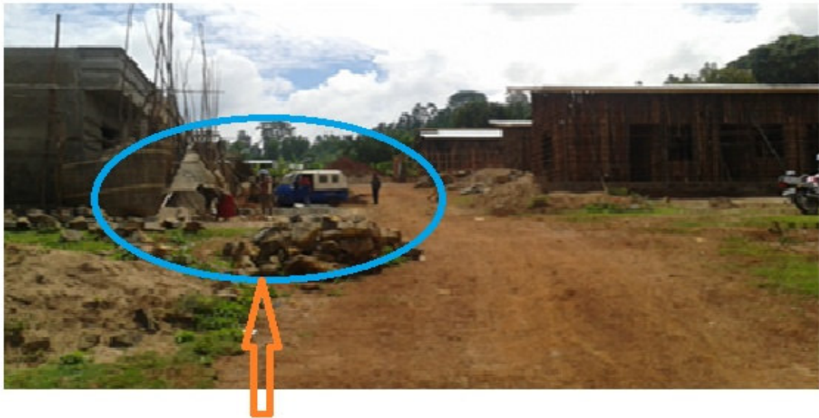
Road narrows as site development encroachment on it.
