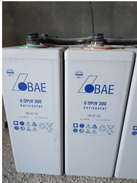
Figure 3. OPzV Battery Used in System
