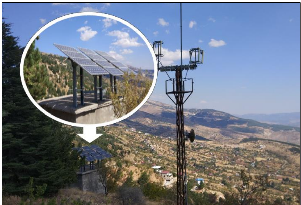
Figure 2. Solar Powered Telecommunication Station located in Sulutarla, Kahramanmaraş
