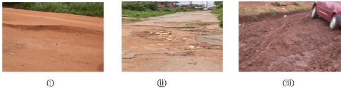
Figure 1. Failed sections of pavements in Akure, adjacent to sampling points (i) S1 (ii) S2 (iii) S3
