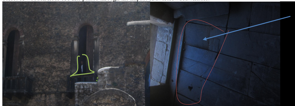
Fig. 12(A), a person standing on the historical wooden structure to have a photo at the back side of the castle of Fasil and (B), the wooden floor of Fasil palace and the circle show the defect of the floor.
