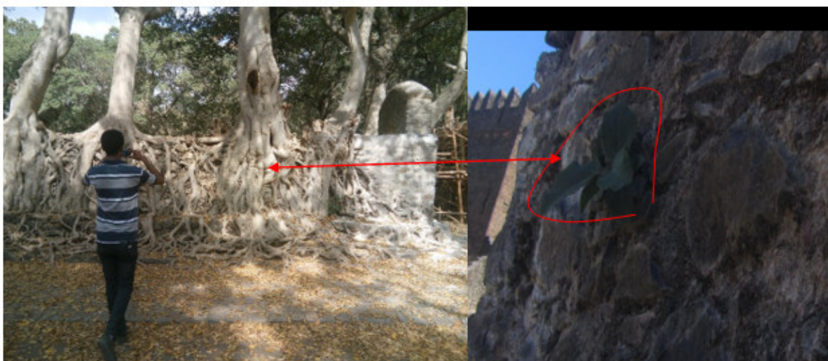
Fig.8 the structure destructed by big trees at Fasil bath and a small tree growing on the left side of the stair goes to the second floor of Fasil palace (Photo by the researcher, January 2019).
