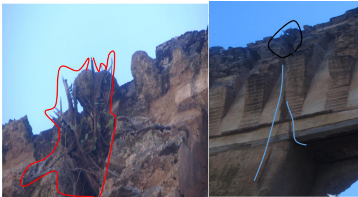
Fig. 1(A), shows the tree grown on the upper and internal wall of the structure at the southeastern facade of AdiamSegedEyasu's Palace and (B), shows how much the root of the tree (shown at A) go down externally and we can estimate the other part of the root is go deep inside the structure to this much (Photo by the researcher, December 2018).
