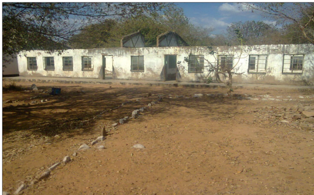
Figure 1 Luunga primary school classroom block-roof blown off by wind in 2006 and not yet roofed to date
