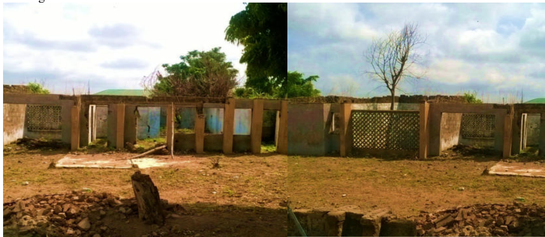
Plate 1: Uncompleted and Dilapidated Abandoned Structures in the Odota.
